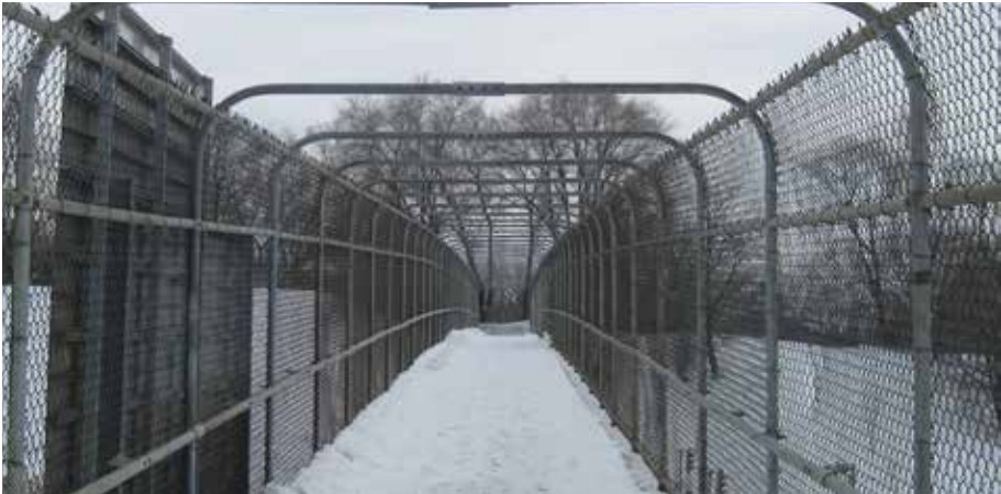
Figure 30: Pedestrian bridge east of Etna Station is located far from main pedestrian activities
