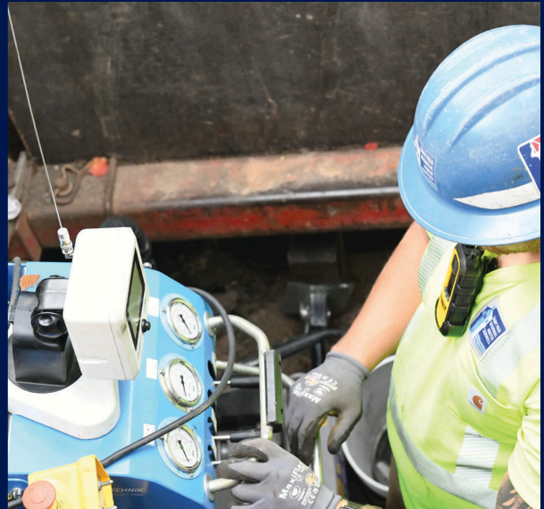
A worker guides a directional boring device through the ground as part of the lead service line replacement process.
