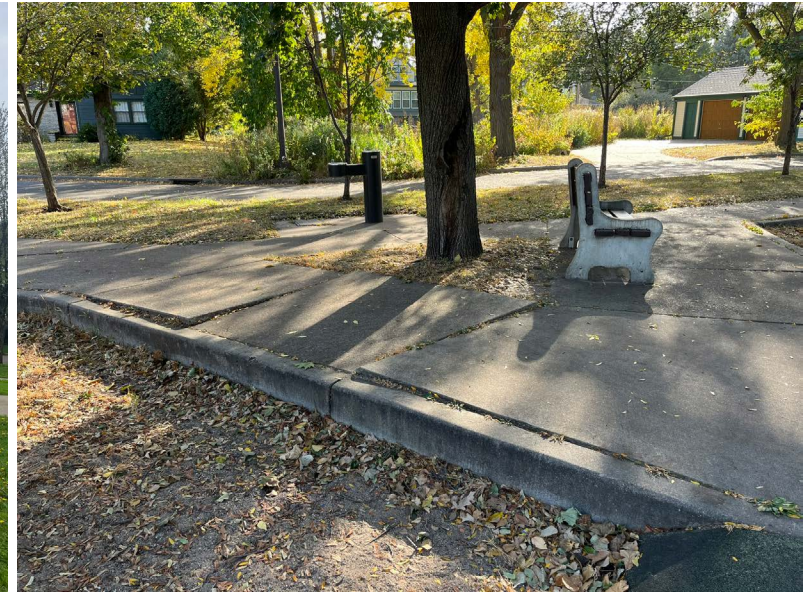
Some pavement in poor condition; impacts from tree roots
