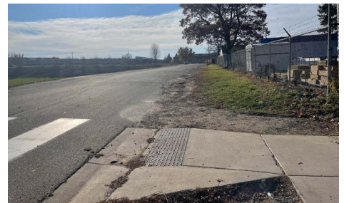
Missing sidewalk connection on Beulah Ln
