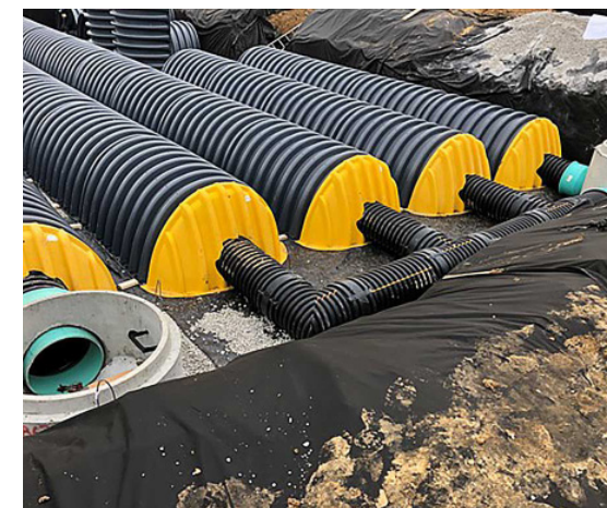
B : UNDERGROUND STORAGE Highly impervious light industrial and residential sites may use underground storage methods to effectively manage the sites' stormwater loads.
