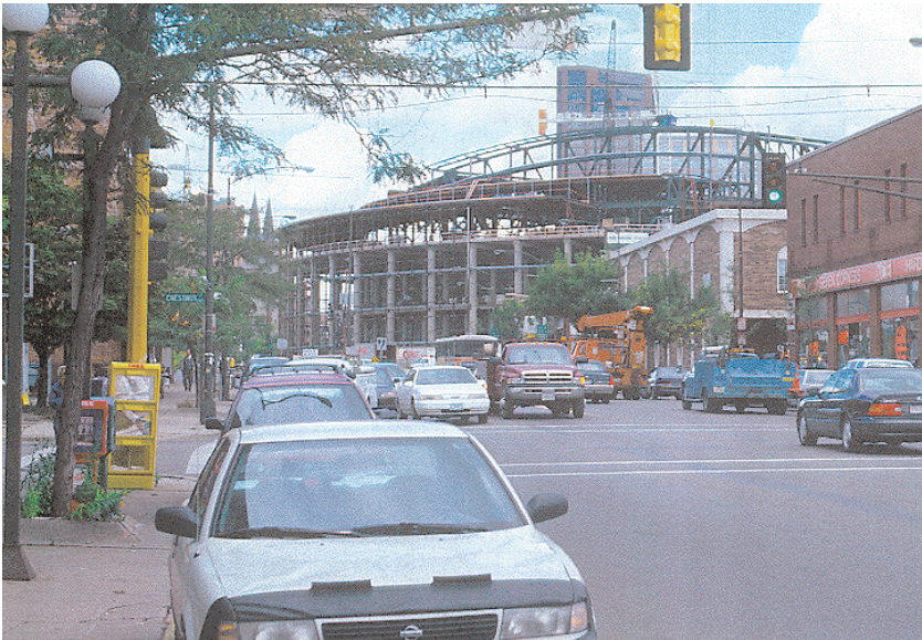
The new arena under construction at the east end of West Seventh Street.
