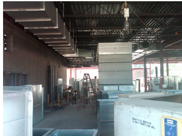
Ductwork and supplies.
