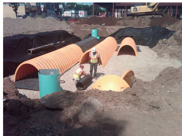
Stormwater drain structures.
