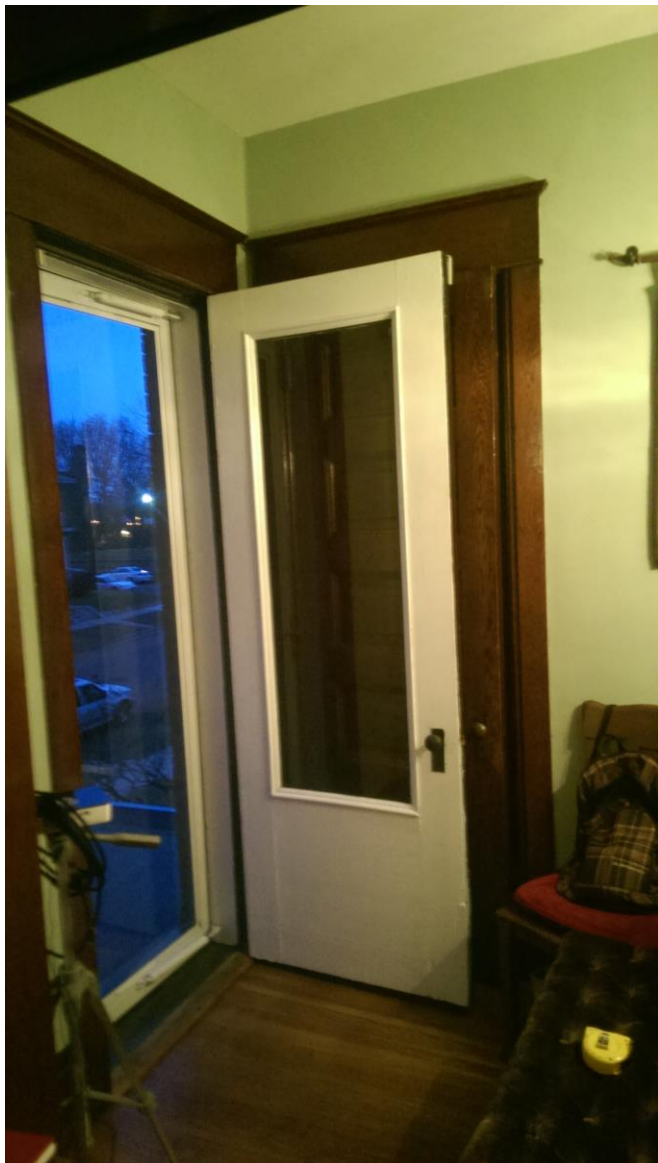
Interior Door, note Casing match Closet Height
