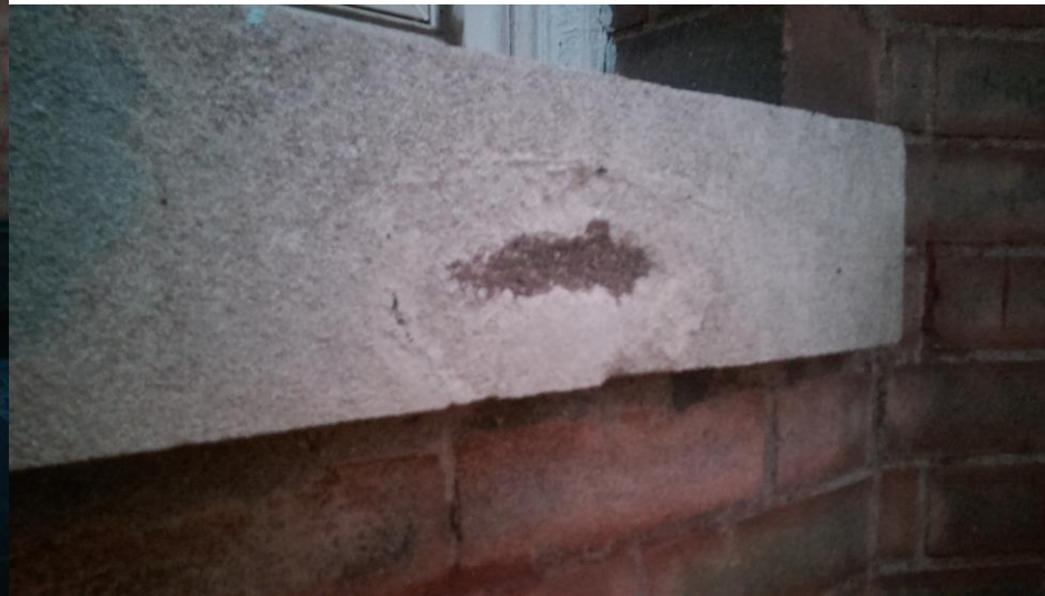
Close-up of the east side where sandstone eroded around original railing
