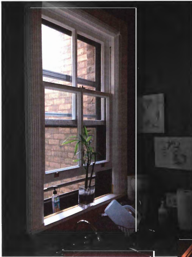
Kitchen window. Full divided light 2 over 2. Proposal to remove this feature, other units in the building do not have this feature.
