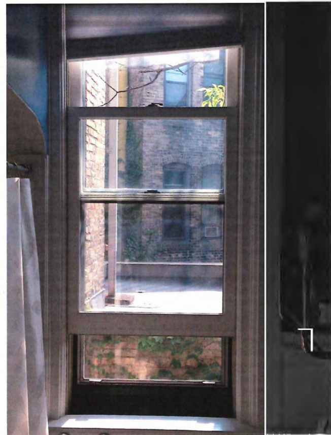
Bathroom window. Clear glass. Out of square. 80's jamb liner (pictured on later slide)
