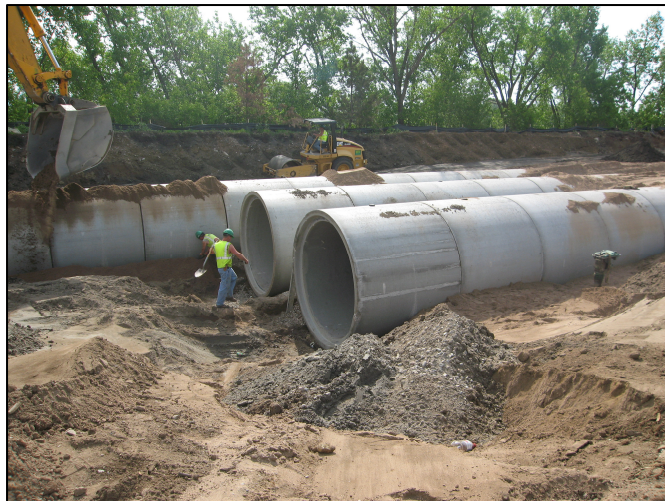
Underground storage can be used for infiltration or storage for potential stormwater reuse, as was done by American Iron in their metal scrapping processes. Project by Barr.
