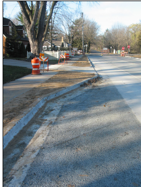
Porous pavement used in parking bumpouts to treat stormwater in Minneapolis. Project by Barr. Photo Credit: E. Holt
