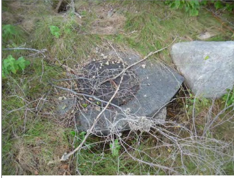
Photo 11: Remains of storm water catch basin at E Indian Ave and Custer St.
