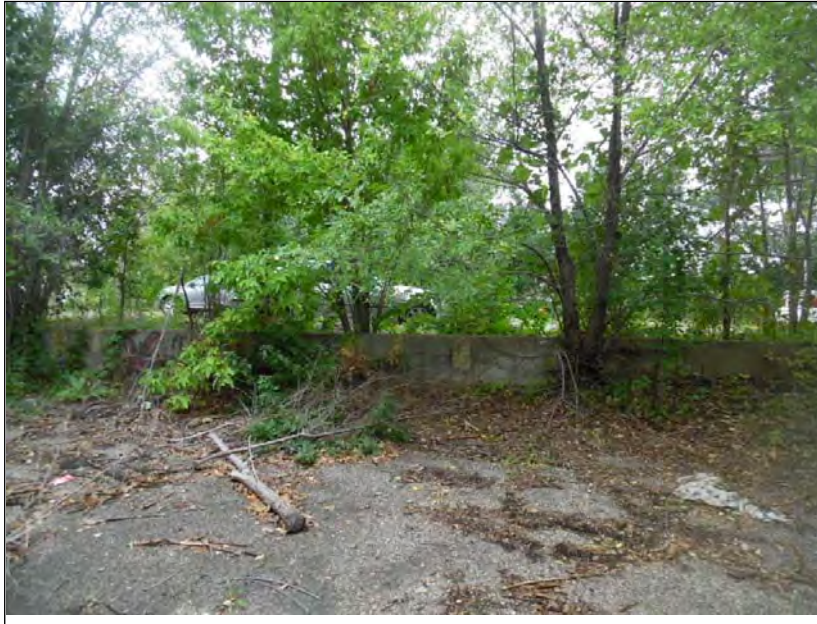
Photo 7: Remaining wall and parking surface along E Fillmore Ave
