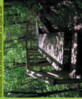
Boardwalk with eroded condition on uphill side.
