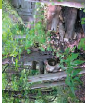
Severely eroded promontory.
