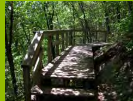
Boardwalk with eroded condition on uphill side.
