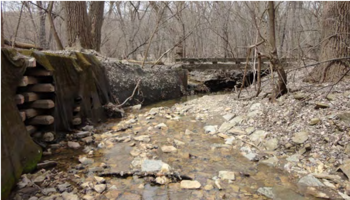
Figure 23: Alluvial Fan Reach - Bank erosion project on channel left looking downstream at Station 6+00 to bridge #2 crossing
