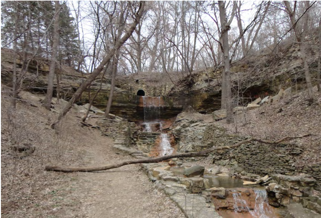
Figure 6: View of Hidden Falls showing the worn and undercut Platteville Limestone caprock, fallen limestone blocks and existing pools and cascades of upper falls
