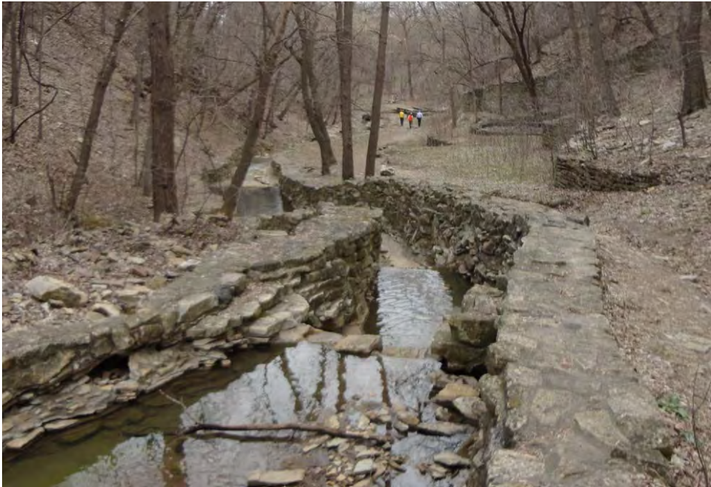
Figure 18: Upper Step Pool Reach looking downstream through the walls of the upper cascades and the ravine valley
