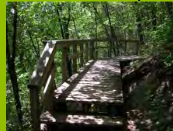
Boardwalk with eroded condition on uphill side.
