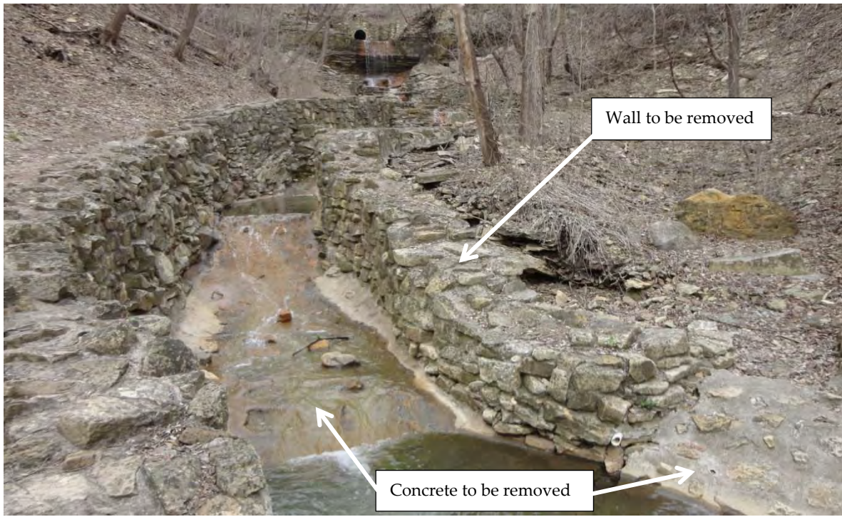
Figure 33 – East wall and concrete lining should be removed in the upper step pool reach.
