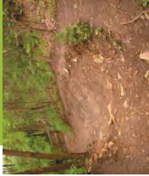
Sloped and eroded trail, where wide stairs are recommended.
