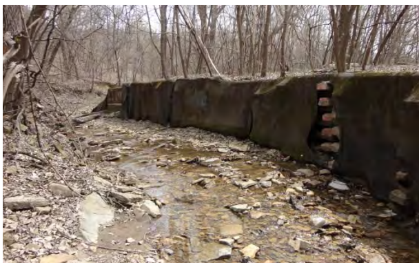
Figure 41: Existing bank armor to be removed.
