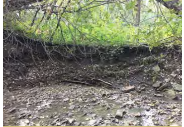
Figure 2.3: Bank erosion from Hidden Falls storm outflow
