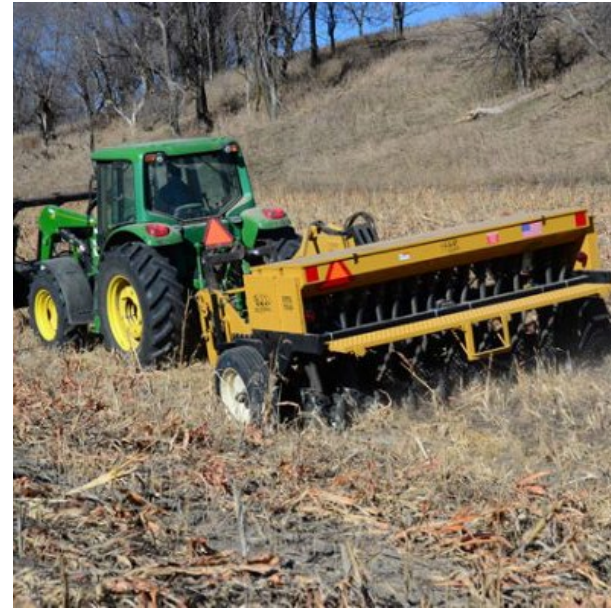
INSTALL Drill into sprayed turf with little to no soil disturbance (2" drill)- Light Harrow if needed in areas inaccessible to Drill
